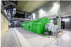
3 000 MVA short-circuit generator
