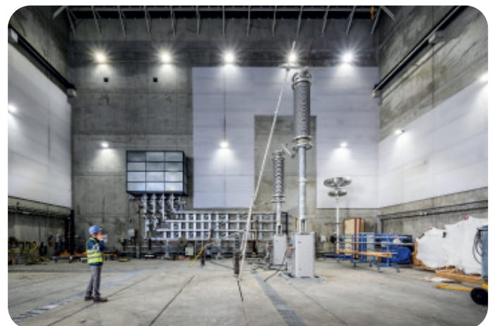
The High Power Short-Circuit test platform - 25m (L) x 25m (W) x 25m (H).
