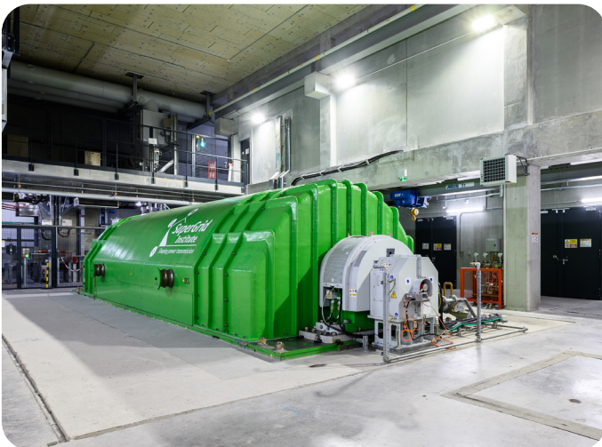
The 3000 MVA generator.
