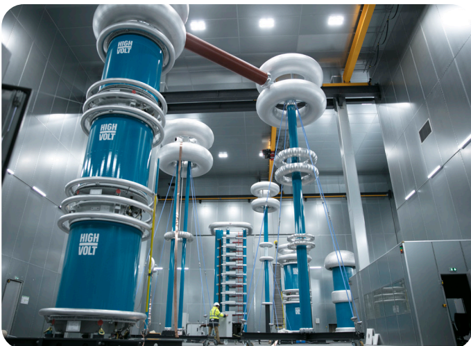
SuperGrid Institute's High Voltage test platform.
